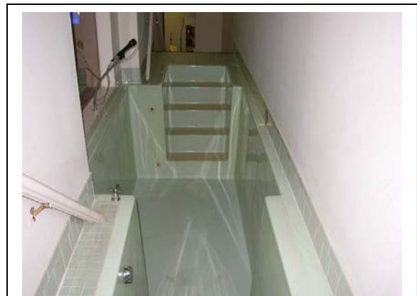
This photo illustrates a corded microphone installed in the baptistry. The risk of electrocution is present for anyone in the baptistry who could contact the microphone. The microphone in this photo should be relocated and suspended from the ceiling or replaced with a cordless microphone.
