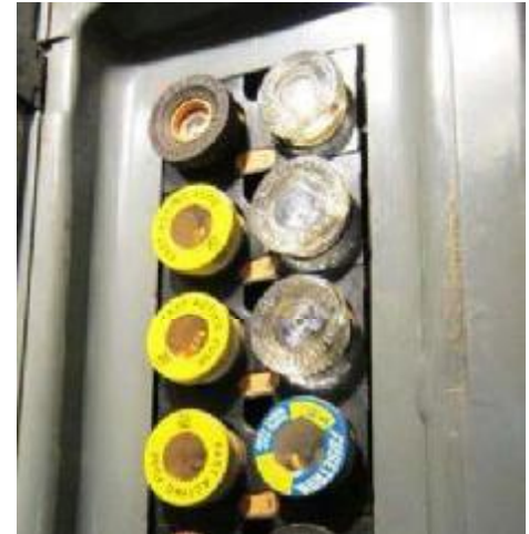
Typical screw-in fuse panel.
