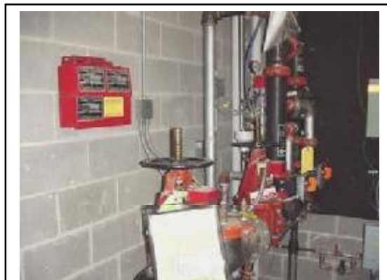
This photo is an example of a sprinkler system main valve. Note the inspection report attached to the sprinkler main. The report will contain information on the sprinkler system, when it was last inspected, and details regarding the inspection.
