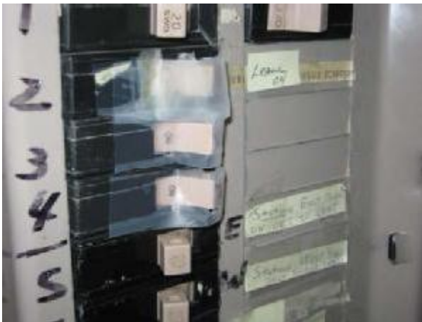
Image above shows breakers taped in the ON position. This practice should never be done.
