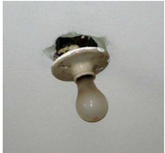
This image shows a light fixture that is unsupported, which puts undue stress on the electrical connections.
