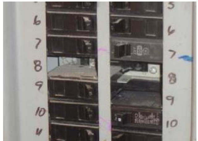
Image above shows open spaces in the electrical panel. Spare clips should be installed in these spaces.
