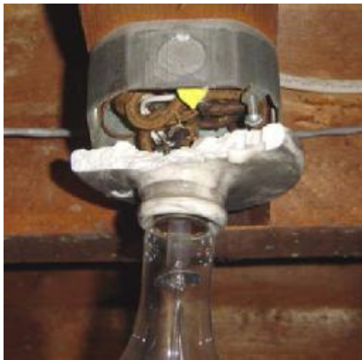
This image shows a broken light fixture. This exposes the wiring to physical damage, dust, dirt and moisture accumulation.
