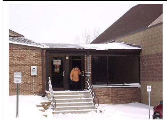
The potential for a severe injury resulting from a slip and fall from the snow-covered steps and landing is high. This demonstrates the need to act quickly to remove snow and ice from walking surfaces.
