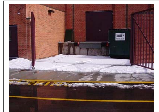
This photo illustrates how melting of snow from a loading dock can cause ice conditions to develop on walking surfaces.
