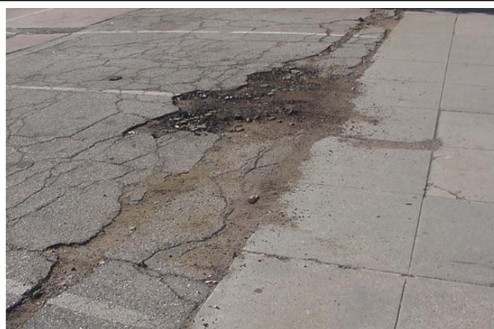
This photo illustrates a parking lot that has deteriorated creating trip and fall hazards due to the numerous cracks and depressions in the surface. To correct this hazard, the sections of asphalt should be resurfaced.
