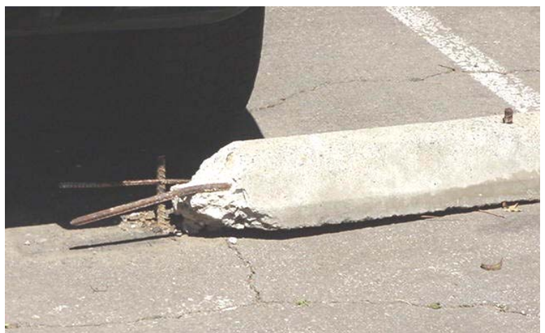
This photo illustrates a severe trip hazard due to the exposed rebar from the deteriorated tire stop. If a trip and fall would occur here, the potential for a severe injury is present from the sharp and exposed rebar rods. To correct the hazard, the entire tire stop should be replaced.
