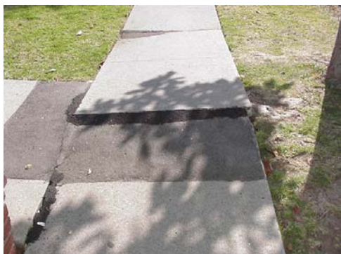
This photo illustrates severe trip hazards due to the uneven walking surface. Patching has been completed; however, it is not adequate. In this case, the entire section of the sidewalk should be replaced.
