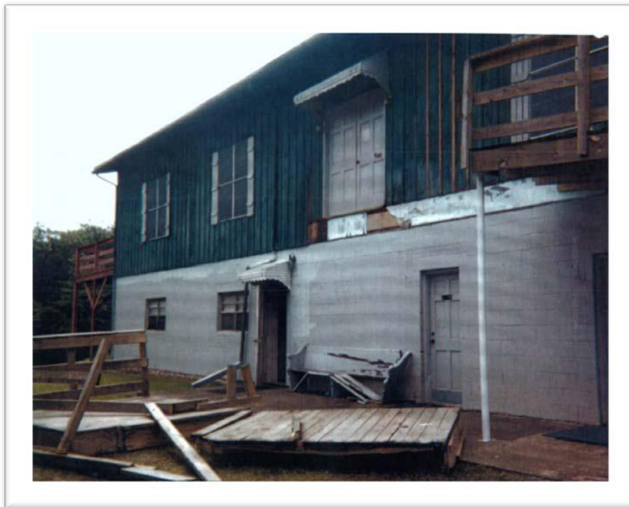
The photo shown here was taken after the accident. Note the complete collapse of the wood deck to the ground and the distance of the fall.
