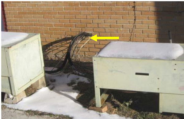
Image above shows an inadequate wiring set up for the central air conditioning units. Electrical is wired directly to the A/C condensing units, without a safety disconnect.
