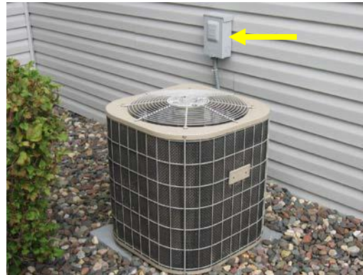
Image above shows the correct installation of an electrical safety disconnect switch.
