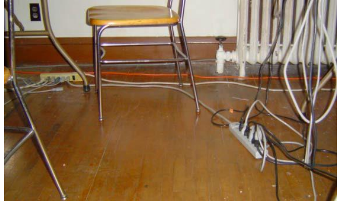
This image shows two power strips that have been plugged into each other, also called daisy chaining. This practice should not be permitted.
