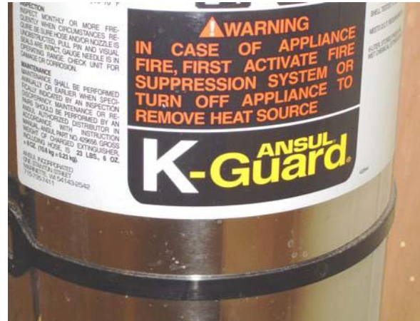
This is an example of a Class K fire extinguisher. Note the warning to only use after suppression system has been activated.
