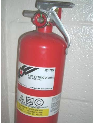
This is an example of a Class ABC multi-purpose rated fire extinguisher.
