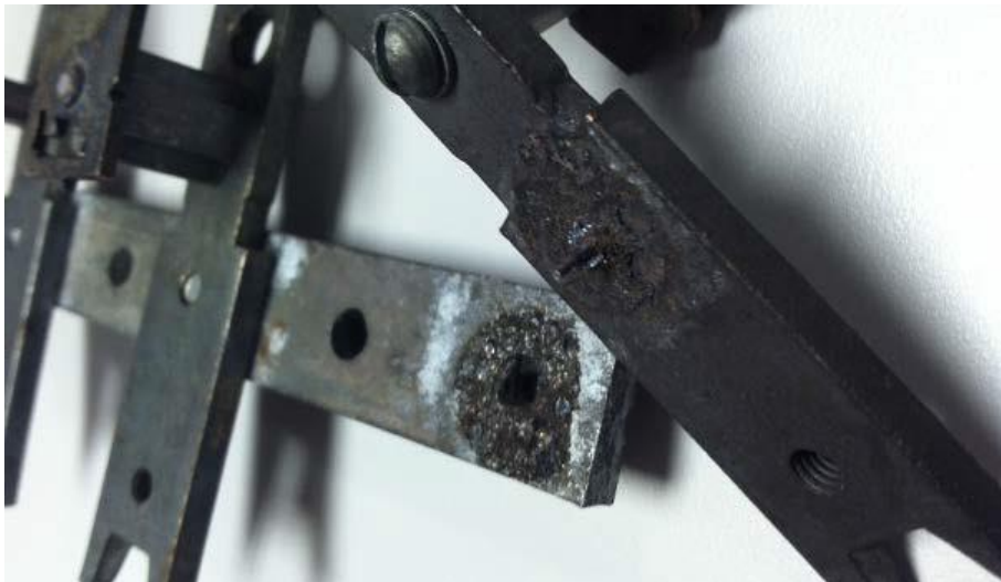
This is a failed, high-resistance, busbar connection inside a 200 ampere Stab-Lok panel. The arced-away steel screw holds the copper bar in the forefront to the aluminum bar in the background.
