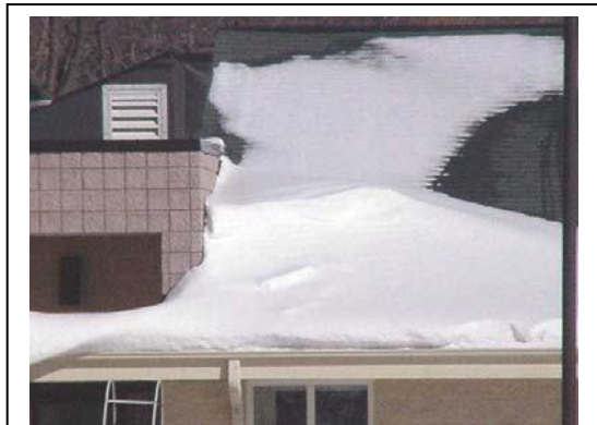
The heavy accumulation of snow on the roof could lead to the formation of an ice dam. Snow should be removed two to three feet from the roof edge.
