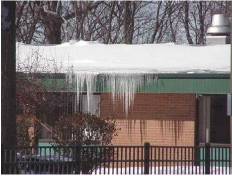
The formation of icicles is a good indicator that there is poor insulation/venting in the attic area. This can lead to water damage.
