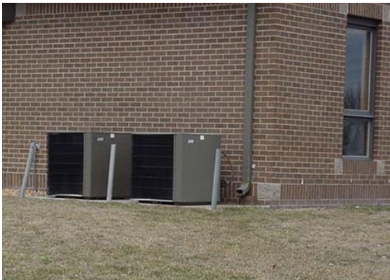
Example: This photograph illustrates AC units located at the back of the building creating an easy target for theft.
