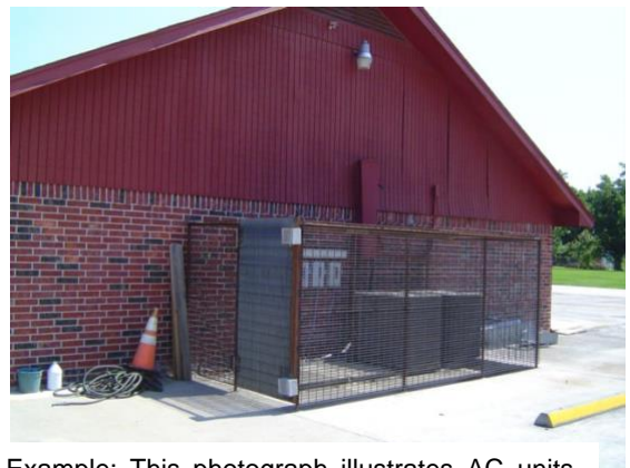
Example: This photograph illustrates AC units protected by a steel cage and security lighting.
