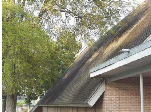
This photo is an example of a tree that should be trimmed back to prevent damage to the roof. Over time, the tree could eventually rub a hole in the roof, allowing water to penetrate the building.
