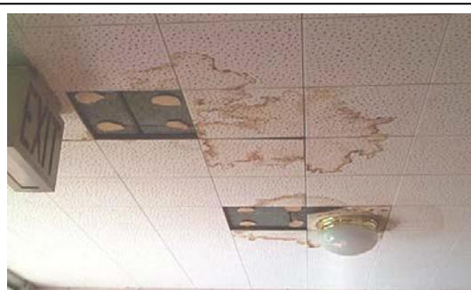
A stained ceiling indicates that water damage has occurred. The source of the water damage should be found and appropriate repairs made.
