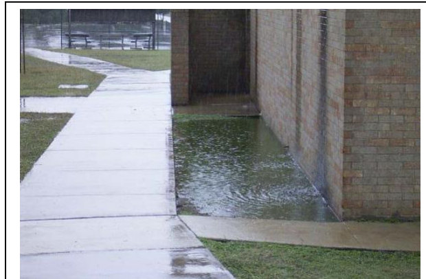
This photo shows inadequate slope and drainage around the building's foundation. Allowing water to settle around the base of the foundation can cause serious water damage to the basement/foundation of the building.
