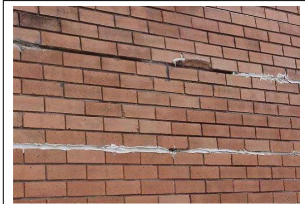
This photo is an example of the wrong way to seal joints in brick. Caulking has been applied to some of the joints. Tuck pointing is needed to repair the mortar joints that have deteriorated by cutting out the old mortar to a uniform depth and placing new mortar in the joints.
