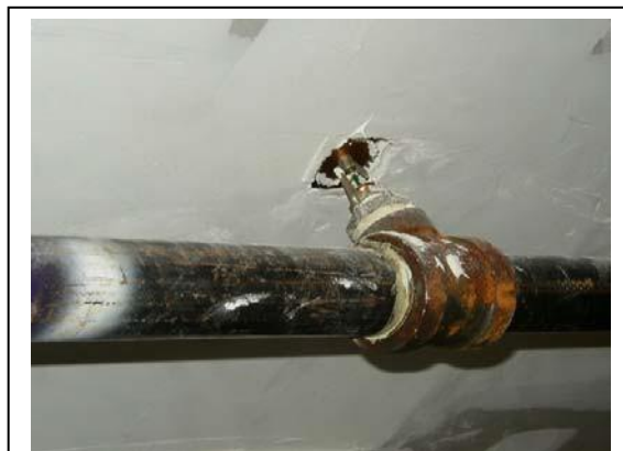
This photo is an example of a sprinkler head that was installed too close to the wall and would not have an adequate spray pattern.
